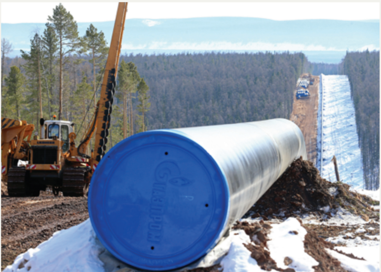
Russia's Power of Siberia gas pipeline to China under construction (source: Caspian News )
